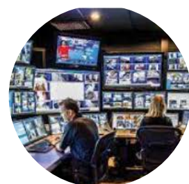
CCTV & Video Surveillance
